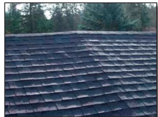
Figure 20-6 Sagging Roof (above 2 images)
