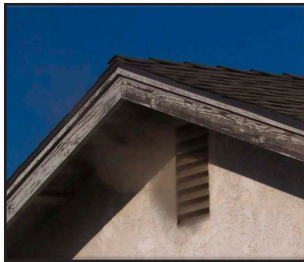
Figure 20-7 A fire in the attic space can compromise roof integrity
