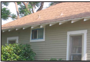
Figure 20-3 The direction and type of rafters can be determined by looking at the exposed eaves
