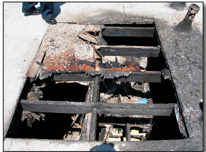
Figure 20-14 Rafter blocking can prevent the roofing material from being louvered and may require the dicing and removal method.
